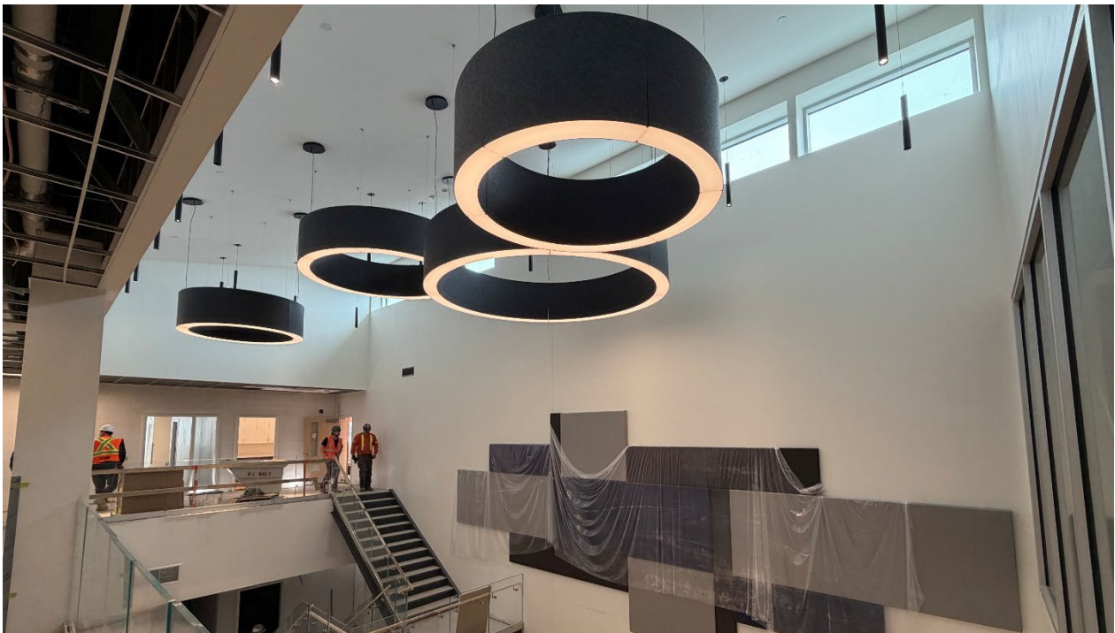
2nd floor, Interior finishing in progress, installation of flooring, ceiling tiles and final coat of paint – March 5, 2026
