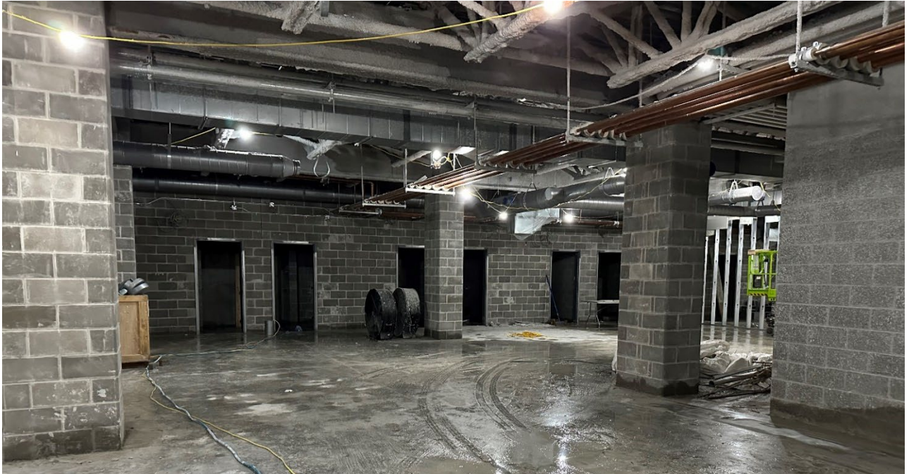
Basement level locker room, masonry walls complete, mechanical and electrical rough in on going – Mar 6, 2025
