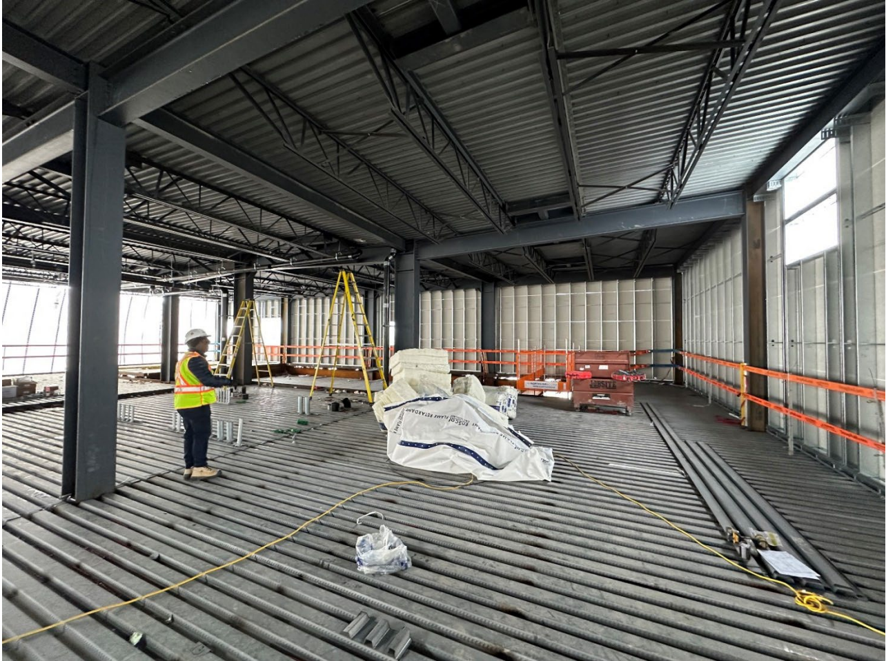
2nd floor, rough in of in floor services in preparation for concrete floor slab pour – Mar 6, 2025
