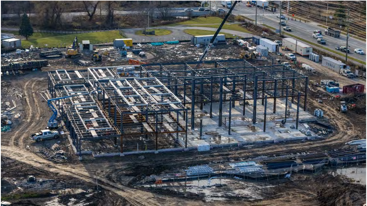
Aerial Photo of structural steel erection, Steeles Ave in back ground – Nov 27, 2024
